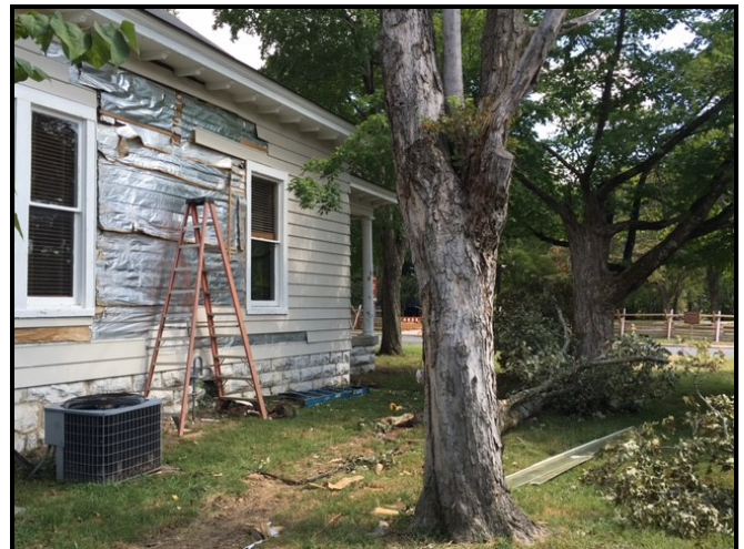
Workmen are clearing trees around the Casa house and preparing the structure for moving.
