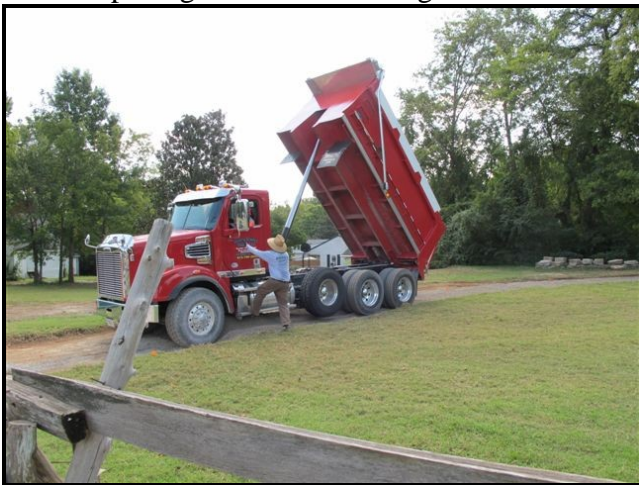
The last of the crushed limestone is dumped for building the trail foundation.
