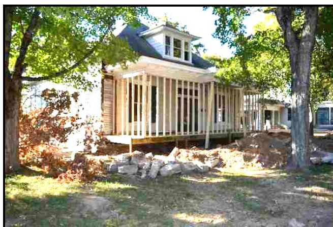
The Casa House, just south of the Carter House, is being prepared for its move to South Hall in Western Williamson County
