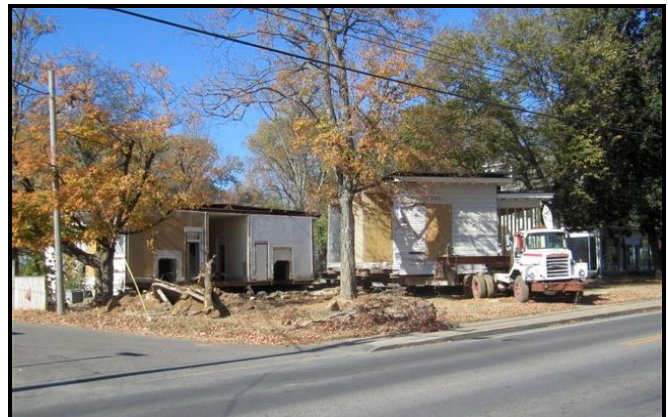
Workmen begin the move of the Casa House section-by-section to its new location on Southall Rd
