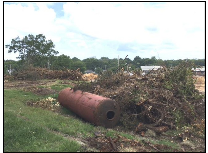
Utilities and trees are being removed from the Old Franklin High School Gym site.
