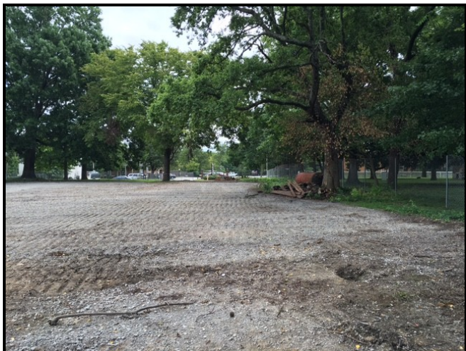
The terrain at the Old Gym site has been leveled to remove the driveways and parking areas. View looking east along the Carter House boundary.
