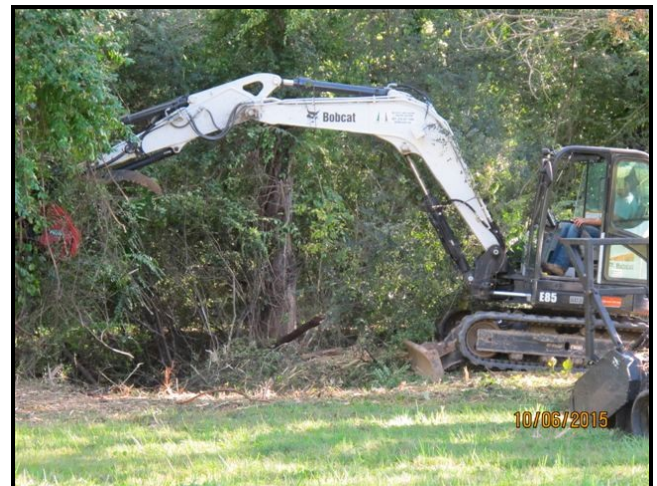
Fig 2. The contractor made short work of briar thickets, privet hedge, and general undergrowth. It was all ground to mulch. Nothing was hauled away.
