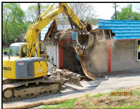
After the pizza party, Ron Crutcher begins the removal of the Dominos building from the Franklin Battlefield
