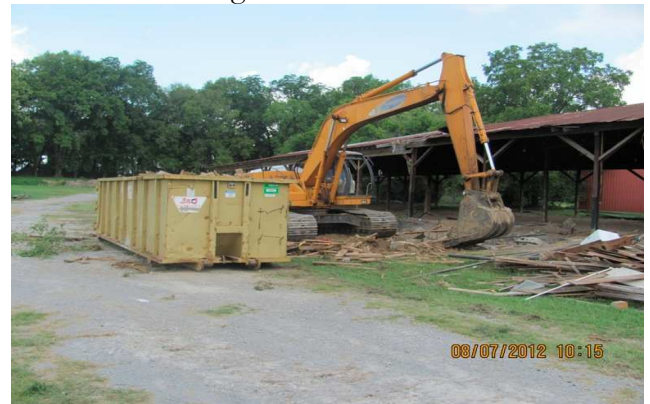
Workmen demolish buildings on Ft Granger parcel. Looking west, Ft Granger can be seen in the tree line
